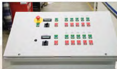
Consolidated electrical enclosure with separate controls for core and laminate
